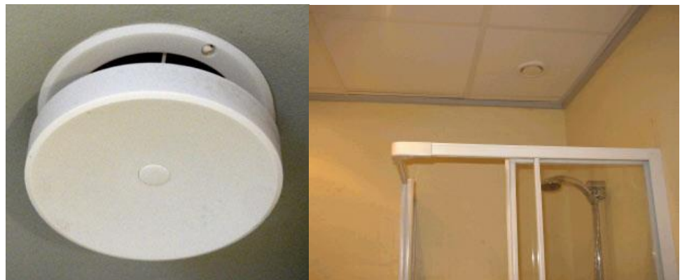
Photo 1 Type of exhaust for mechanical ventilation
